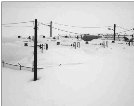
Deep snows blanketed many communities and AVEC's power plant facilities, including this tank farm in Savoonga.
