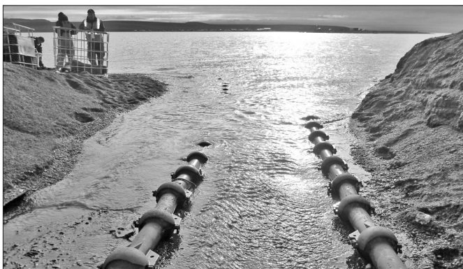
Protective armor covers the cables near the shoreline. The trench was filled.
