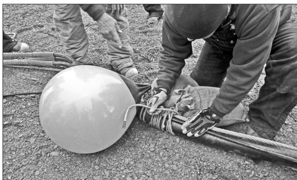
Buoys attached to the cable every 10 feet kept the cable afloat during the pull. Sacks of concrete mix were attached every 20 feet to keep the cable submerged after the floatation buoys were removed.
