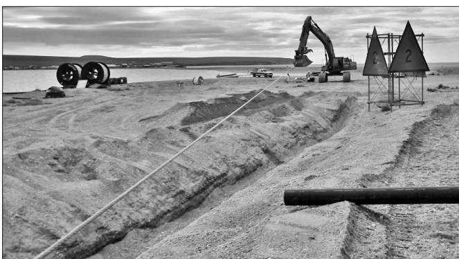
An excavator carefully pulled the tow line and cable into the Teller trench.
