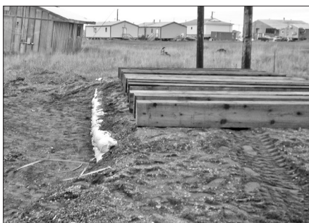
Sturdy wood beams are placed on top of the compacted dirt pad to support the heavy modules.
