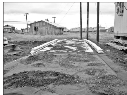
Gravel is poured and compacted on top of the prepared pad foundation.
