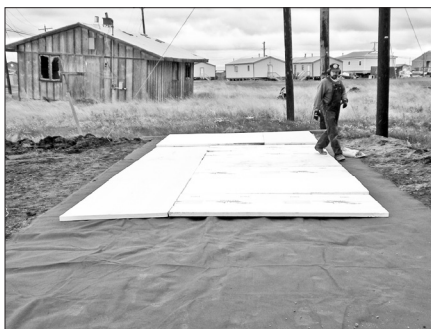
Barry Bryan inspects the insulation used to prevent the ground from thawing.
