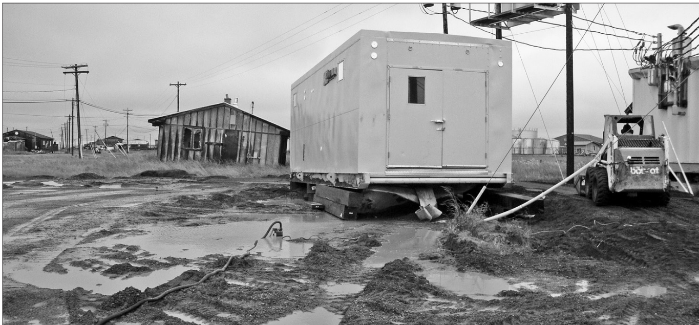
A constant deluge of rain turned the power plant yard into a muddy quagmire that required pumping to drain excess water.
