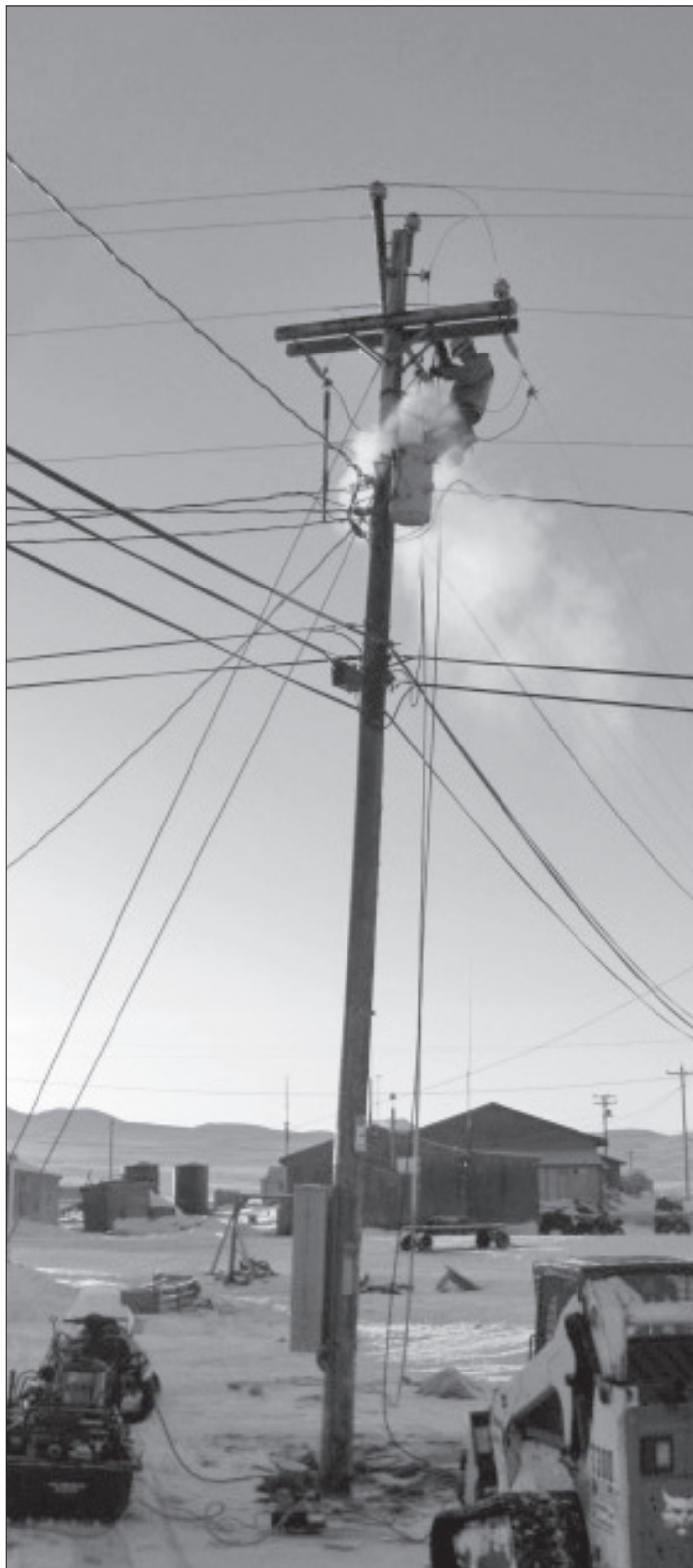
Linemen used a power washer to remove frozen sea-salt spray that coated some power equipment. When asked how he was coping with working in the severe weather conditions, Matt Kruger said, "I'm living the dream!" AVEC's linemen were glad they could help our members and appreciated the numerous "thank yous" received from Savoonga's residents.
