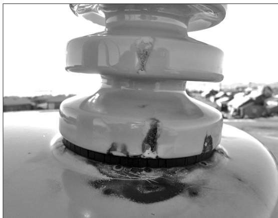
Conductive salt spray caused arcing to burn this transformer and bushing. Burns similar to this occurred on other transformers and bushings, especially those closest to the ocean.
