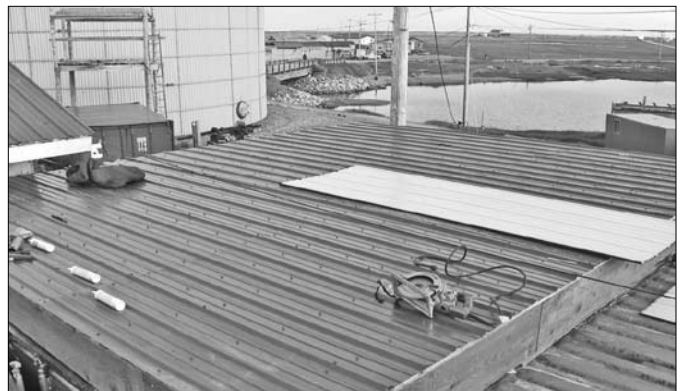
Cutting wood to build the framework and trusses for the new roof, seen below. The roof is anchored so it won't blow away.
