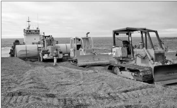
Heavy equipment got stuck offloading and moving the wind tower from the barge.
