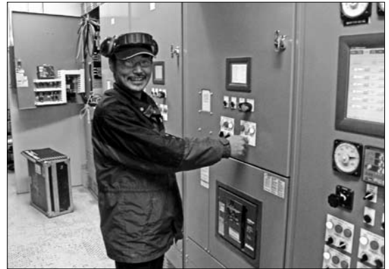
Power plant operator Larry Lake turning on the new control module. Larry is also a certified and talented wind turbine technician.
